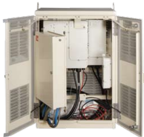
Cross-Connect Service Delivery Distribution Field is Hinged for Easy Access to Feeder or Distribution Cable and DSLAM Protectors.
